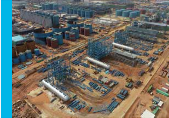
HPAL Autoclave Area
