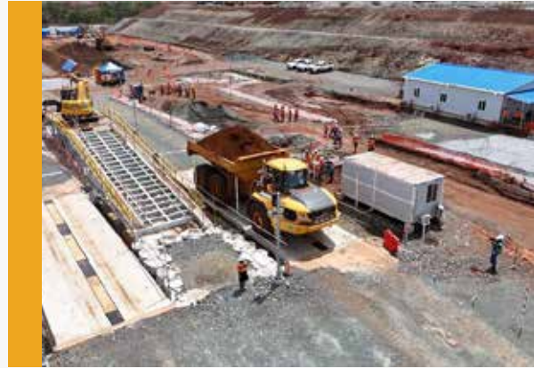
Weighbridge Transfer Point
