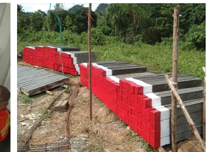
Land border installation
